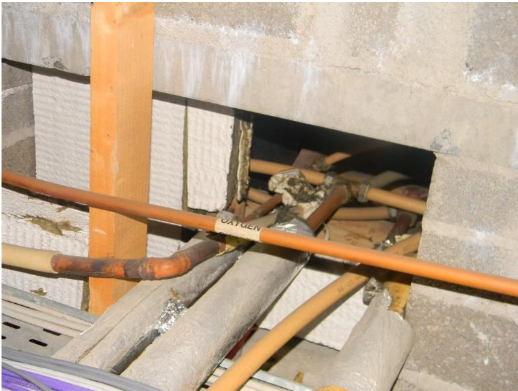
Image 1 - Incomplete fire stopping allowing passage of heat and smoke
