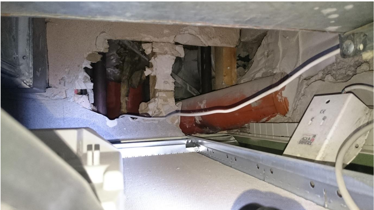
Image 2 - Fire stopping absent allowing the free passage of smoke or heat
